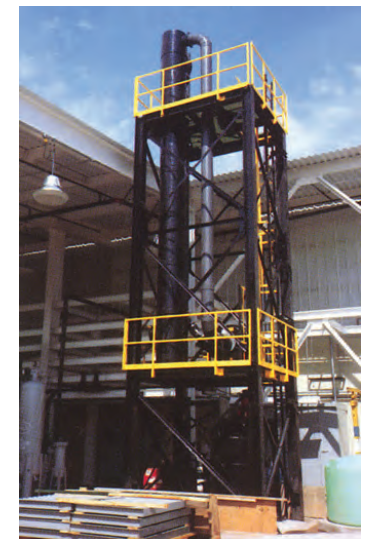
Ammonia odor scrubber
