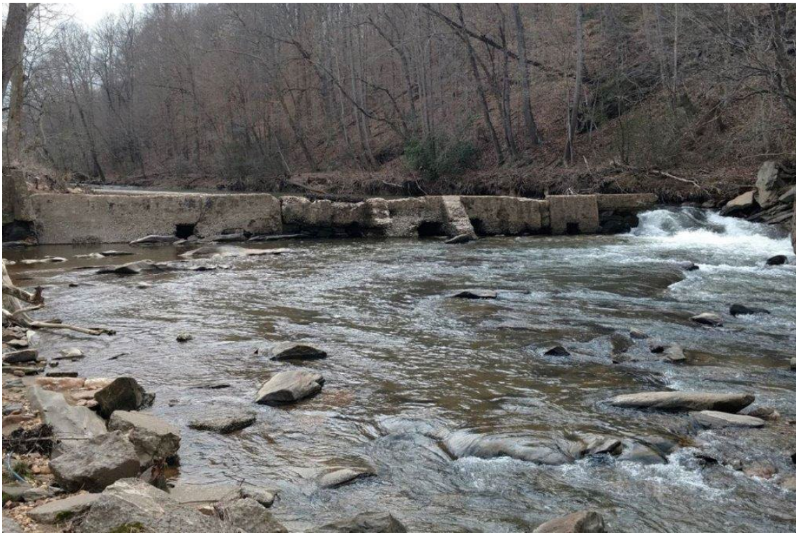
Altice Mill Dam before removal – dangerous breach on river left
