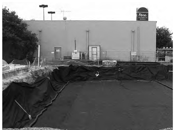
Place non-woven geotextile over prepared soils and up excavation walls. Install underdrains if required.
