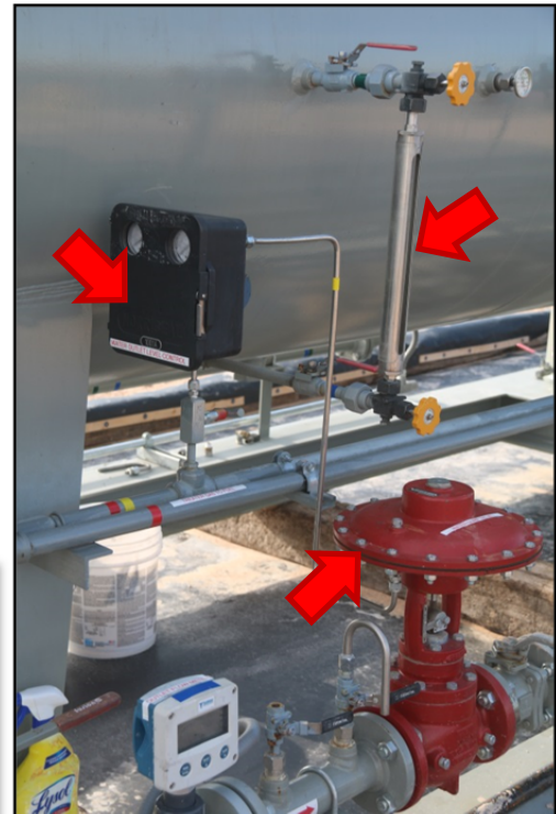
AUTOMATIC SEPARATION VESSEL LEVEL CONTROLS (UNATTENDED SERVICE)
