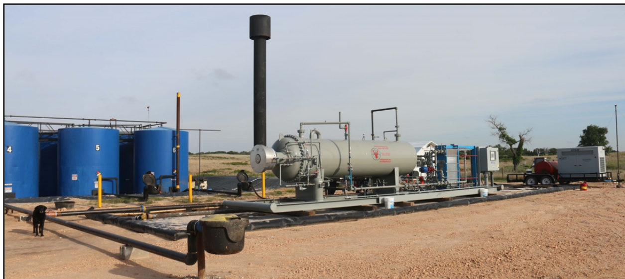
GRAPHIC 1: L-POD ® INSTALLED IN A PIPELINE TERMINAL IN WESTERN OKLAHOMA (5/2015)
