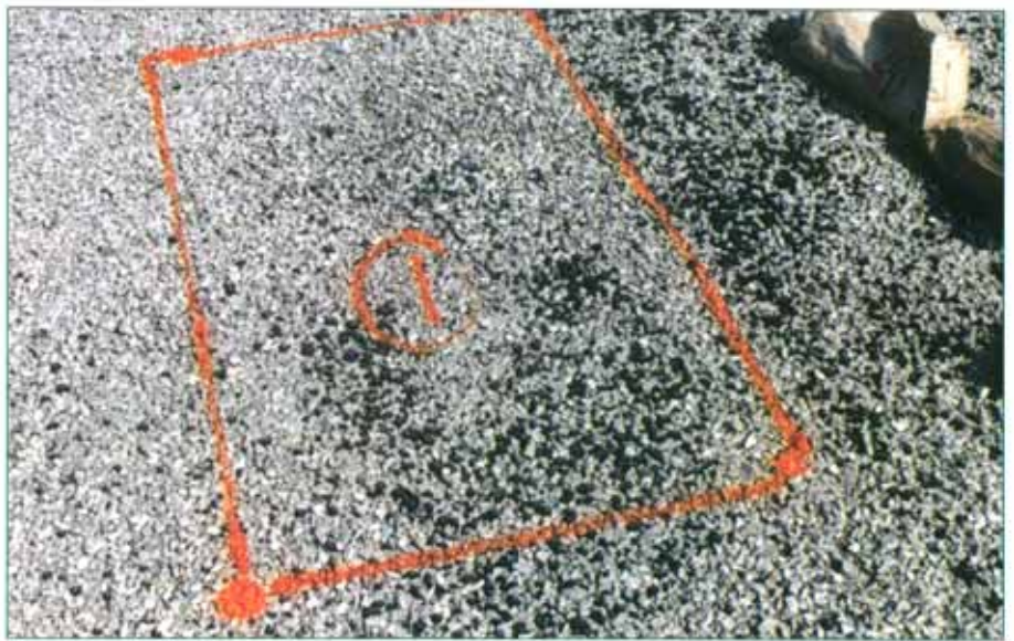
Thermal anomaly denoted on roof
