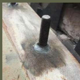
New Clamping Studs & Hardware
