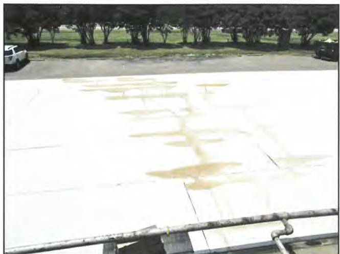
Figure 9 – Stained cap sheet from water draining across sheet.
