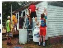
Removing poorly-installed siding
