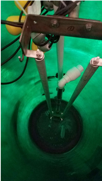
Interior of Pump Basin
