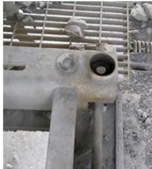
Broken Tension Bolt
