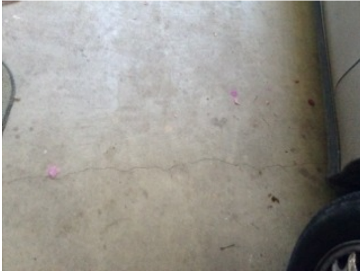
Very minor slab cracking
