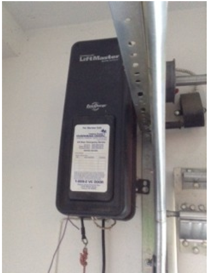
Door motor does have working safety chain
