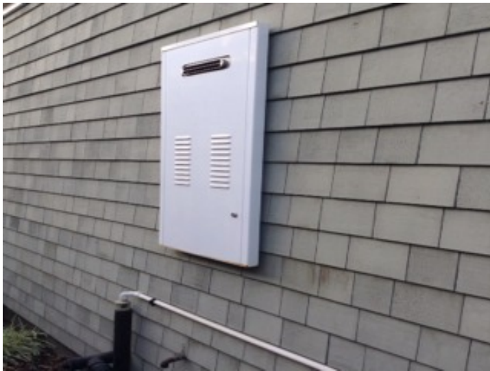
Instant hot water system <5 years old
