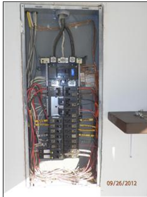
9.6 Picture 1 Breaker Panel
