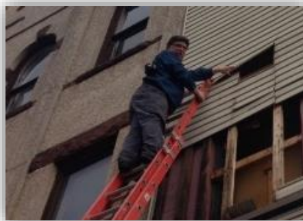
Nick DiPasquale of Spec Restoration removes a portion of the siding obscuring the building's historic brick and window openings.
