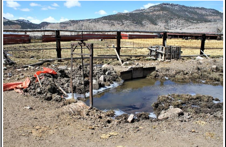
Headgate and overflow gate
