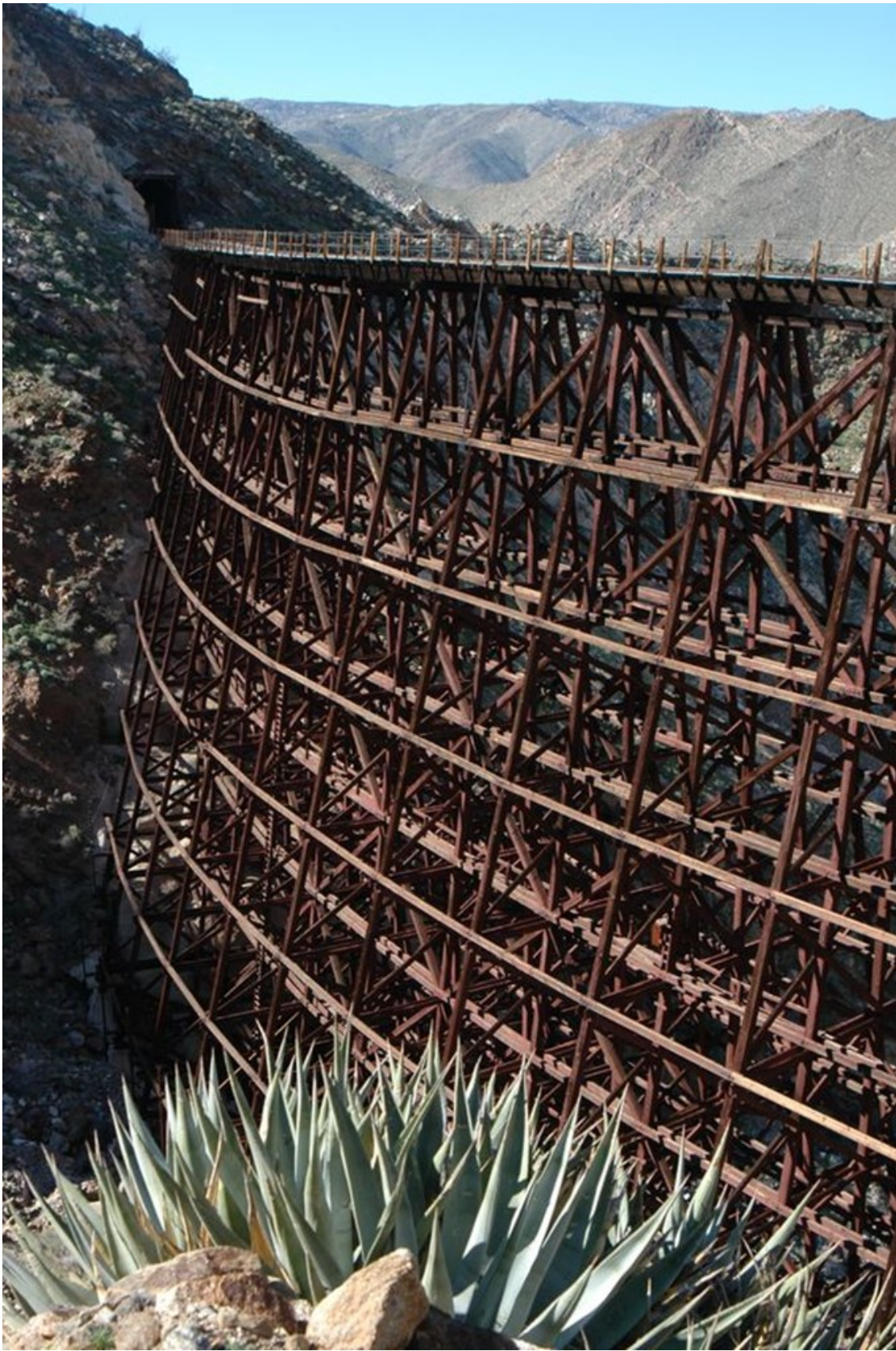
Goat Canyon Trestle built 1932. 750 feet long and 200 feet high. Southern California. The biggest wood trestle in the world. Currently out of service but undergoing repairs.
