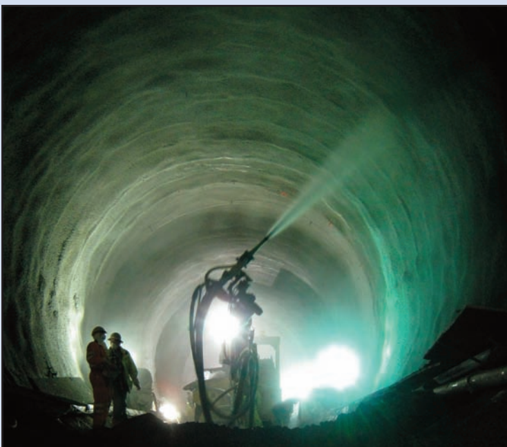
Installation of a smoothing concrete layer is part of the next phase of work. Photo by Frank Jenkins, Dulles Transit Partners
