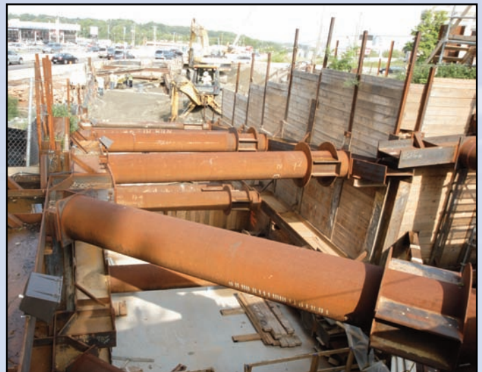
The west end of the cut and cover portion site with westbound Route 7 traffic moving in the background of this photo. Photo by Dulles Corridor Metrorail Project
