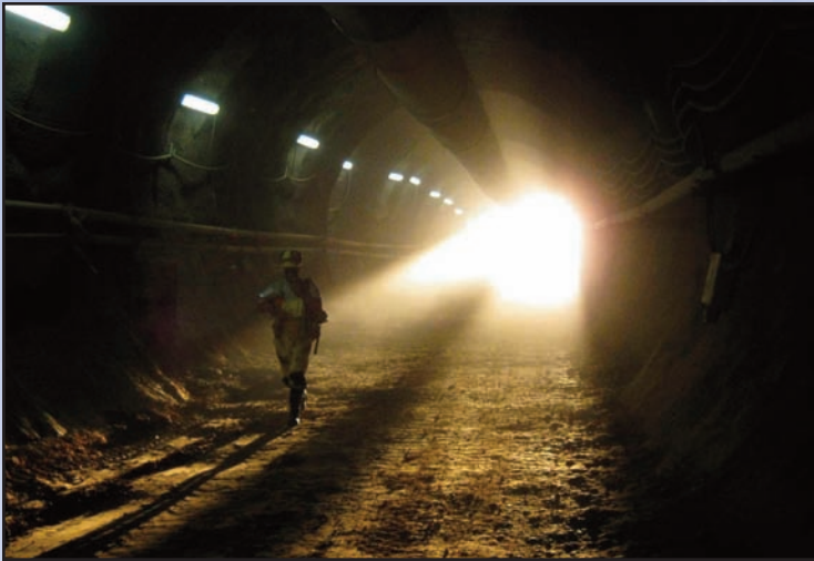
The depth of the two tunnels ranges from seven to 30 feet below the Route 123 and Route 7 intersection near the landmark water and defense towers. Photo by Frank Jenkins, Dulles Transit Partners
