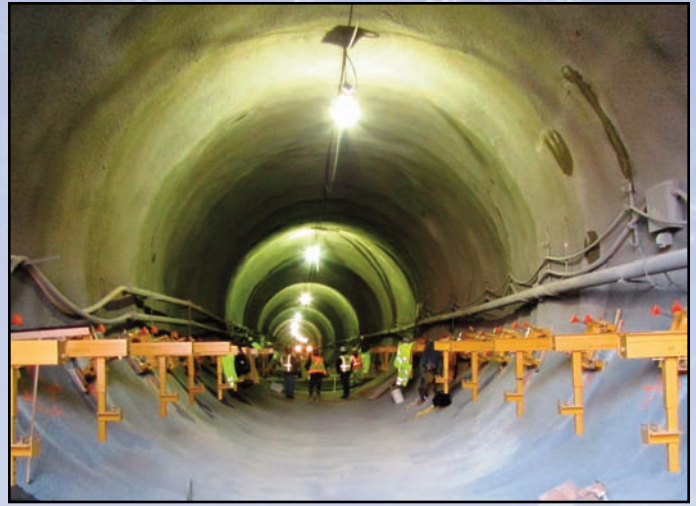
Mining for both inbound and outbound tunnels was completed last year and crews are now providing additional reinforcements. Photo by Dulles Corridor Metrorail Project
