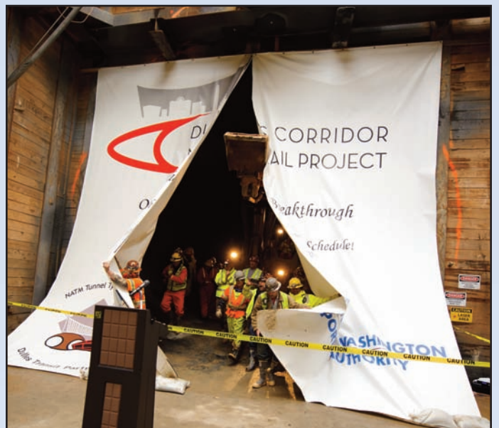
Crews for Dulles Transit Partners, the project's design-build contractor, celebrate the completion of the mining of the outbound tunnel. Photo courtesy of Dulles Transit Partners
