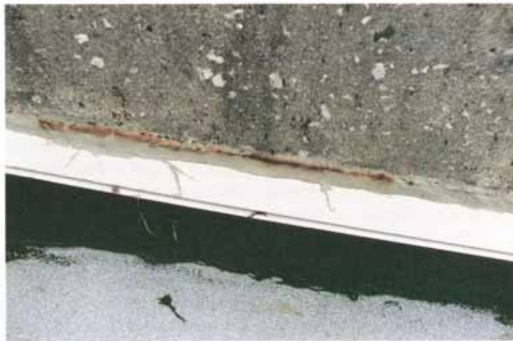
Sealant along caulk trough is contaminated by roofing bitumen.
