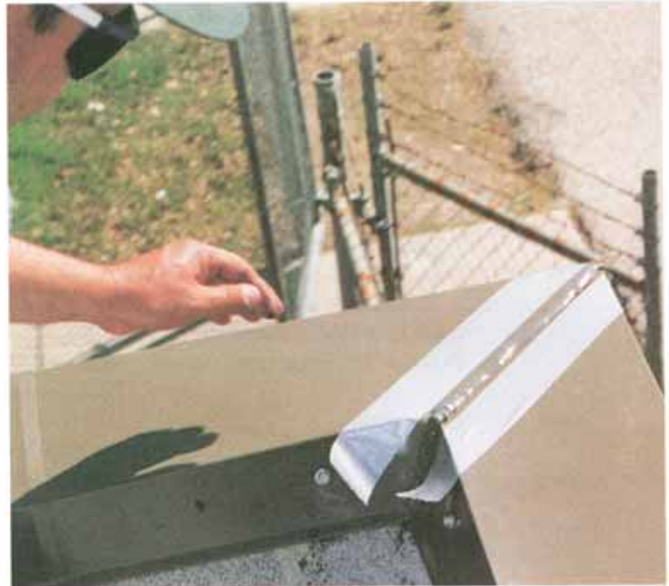
Masked joint: Sealant bead prior to creating cap bead, "band aid" profile.
