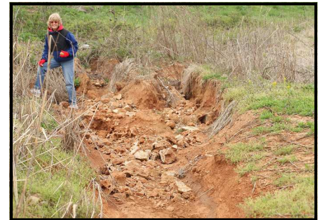
Peg standing on the edge of the washout.
