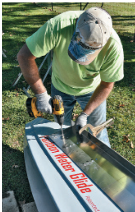
Doug Stewart bolts on the rails that suspend the pod from the deck's crossbeams. The rails are removable, allowing the PWG to be re-installed on another pontoon boat.
