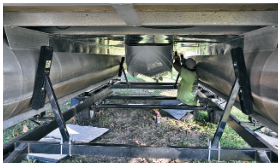
(Below) The PWG pod is secured via the rails to the deck cross beams. This is when an extra hand—or a jack or two—come in handy.
