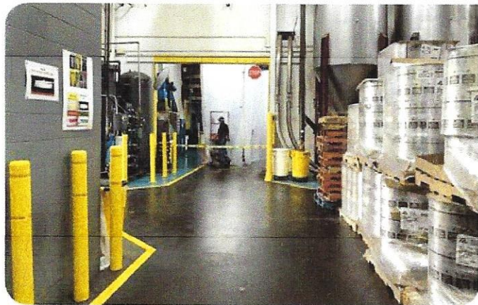
The crew finished with ICO Floor 51/Guard 51 with broadcast aggregate and a layer of ICO Floor Coating/Guard Coating. And with that, the crew was able to call it a day and grab a cup o' joe.
