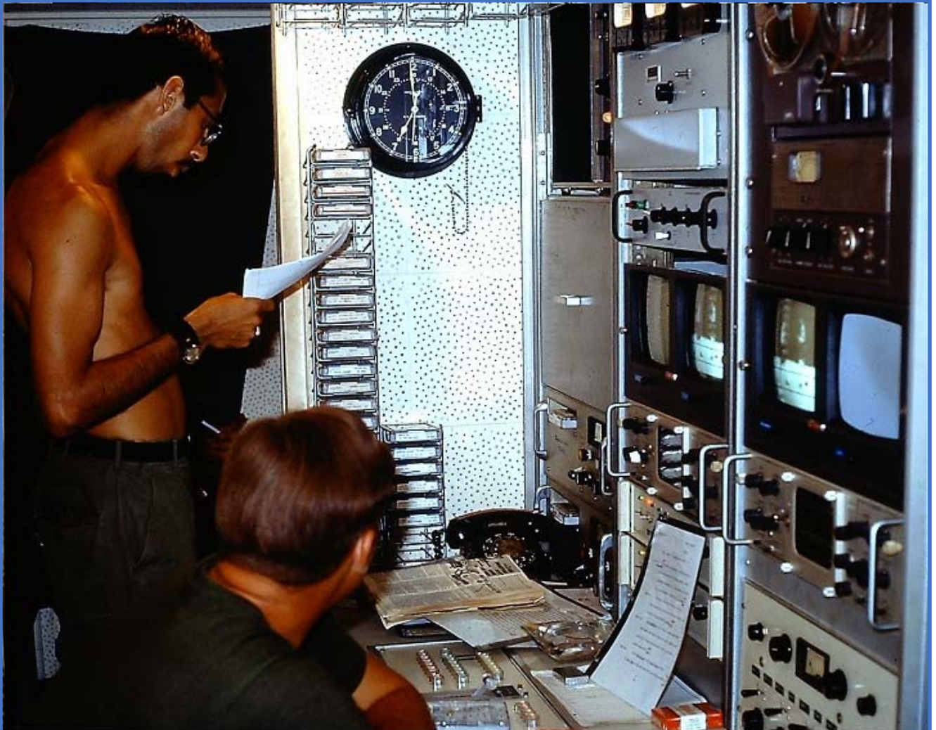
Getting the Master Control Room Ready.
