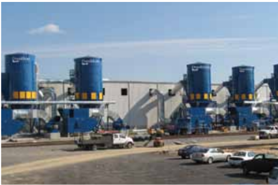
776RF at wood furniture plant
