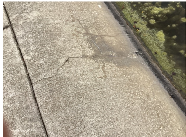
Concrete cracks and spall
