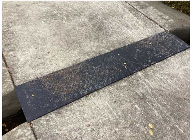
Metal cover rust
