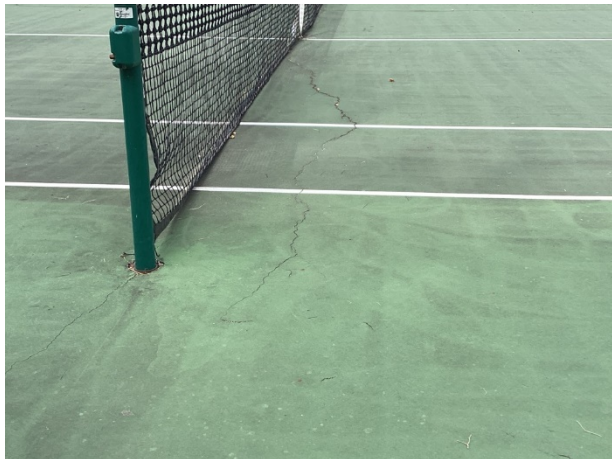
Surface cracks at tennis court
