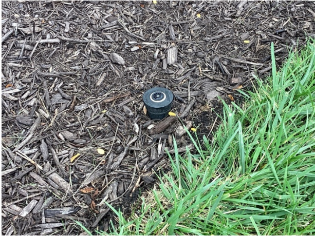
Irrigation system head
