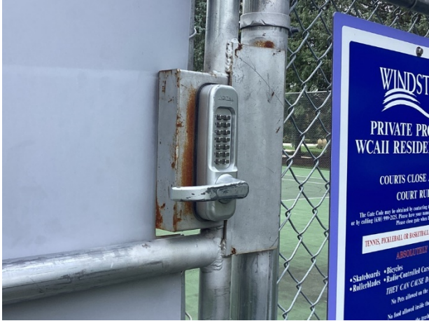
Gate lock rust at tennis court
