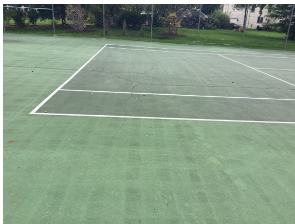
Surface cracks at tennis court
