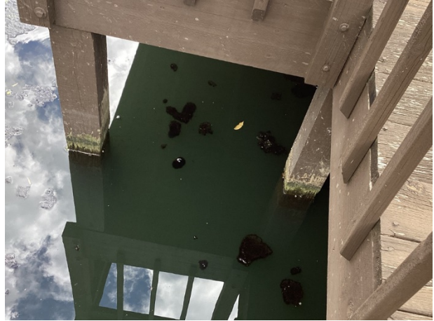
Piling deterioration at large dock
