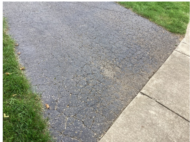
Alligator cracks and raveling
