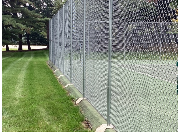
Fence warped webbing at tennis court
