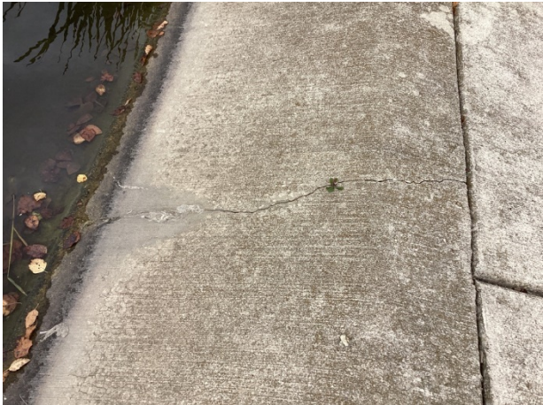
Concrete cracks and spall
