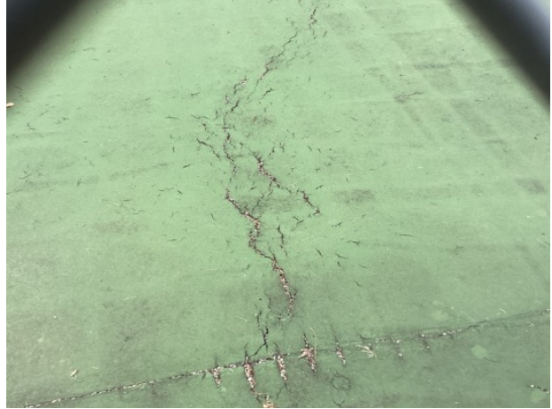
Surface cracks at tennis court
