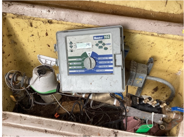
Irrigation system controller
