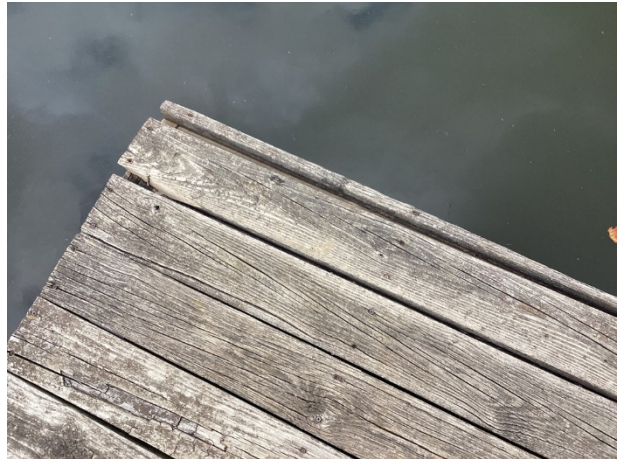
Deck board deflection at small dock
