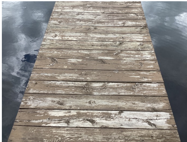
Weathered deck boards at large dock
