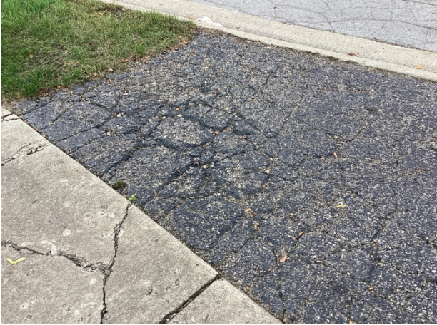
Alligator cracks and raveling
