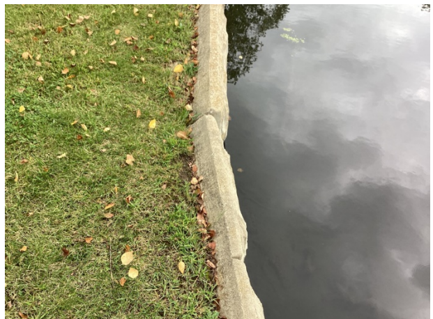
Minor wall movement
