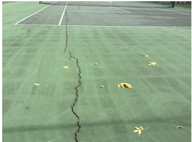
Surface cracks extending across entire length of tennis court
