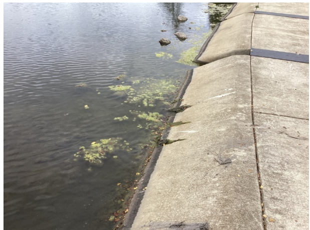
Algae growth at spillway inlet
