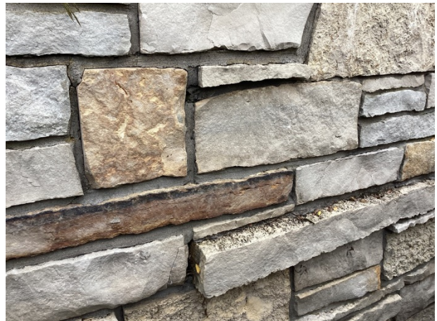
Masonry cracks and mortar deterioration
