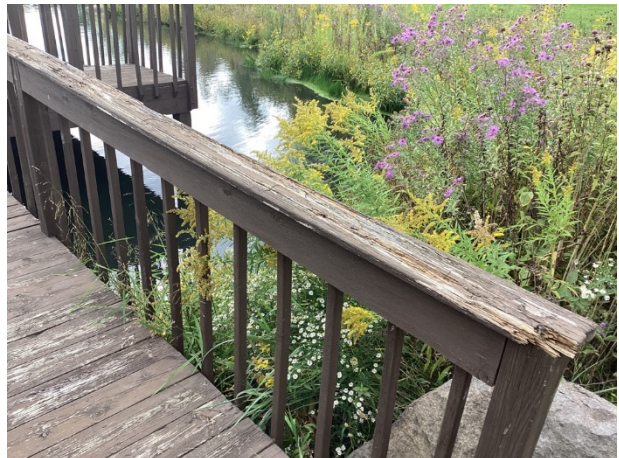
Wood rot at large dock railing
