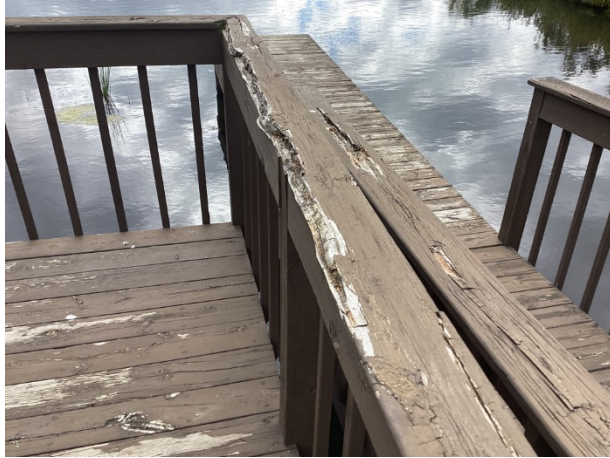
Wood rot at large dock railings
