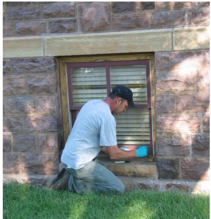
Scott Petersen, windows project contractor, at work on a Carnegie window. September 2010 photo by Lynette Higgins, CRC volunteer.
