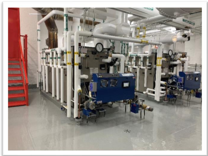
New Boiler (After Design & Installation)
