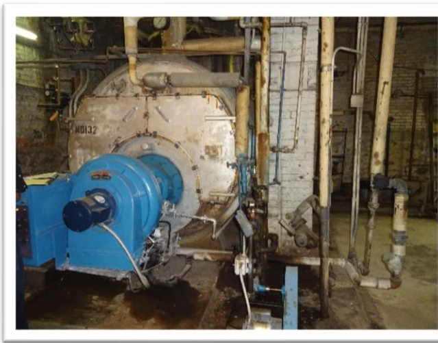
Old boiler (before ECM implementation)
