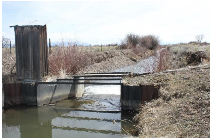
Flume looking downstream
