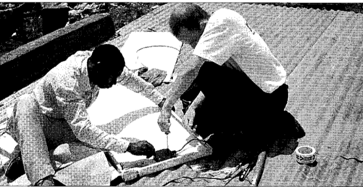
Solar Lighting kits installed
