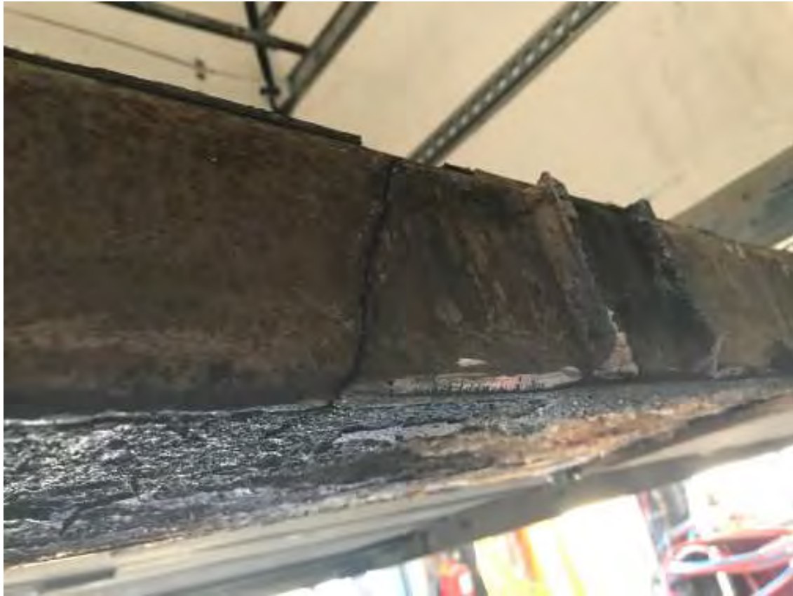
Photo 7 Cracks in crossmember with skid plate removed
