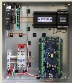
ReMASTER Data Collection System
