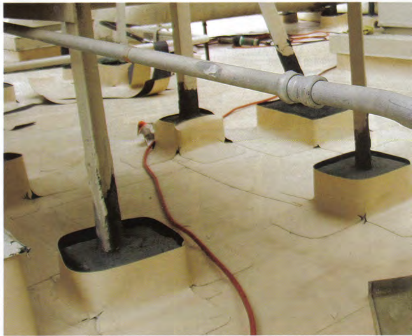
Non-round roof penetrations are extremely difficult to flash. Pitch pockets are the lazy way to encase odd-shaped geometric shapes rather than creating a true roof flashing detail. These examples highlight issues presented by pocket filler products that shrink, crack, and funnel water into a structure. Images courtesy All Style Industries
