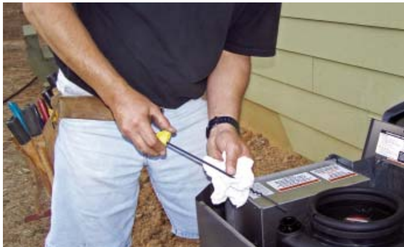
Figure 6. The electrician removes the cover of a 7-kw air-cooled unit and checks the motor's oil level. Air-cooled generators need an oil change after every 50 hours of operation.
