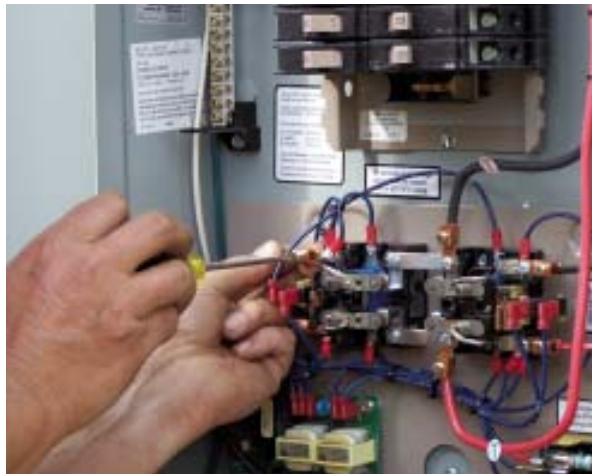
Figure 2. An electrician connects a wire from the main load center to the transfer switch in a panel that contains the load center for the emergency circuits. The thick wires tagged “T” run to the load center above, and the smaller red and black wires on the right go to the generator. The blues are control wires.
