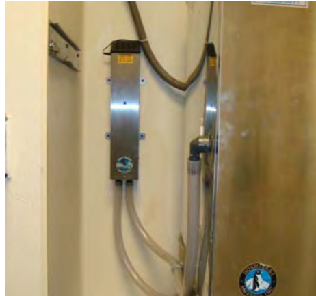
Clean Ice Machine start of testing at Subway Corp.
