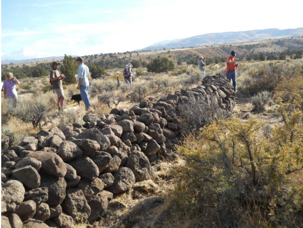
11 people built this rock wall in 2 hours. It was difficult work, even for those in the best of shape.
