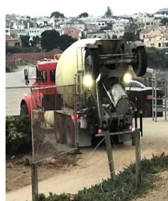
Ready mix concrete truck arrives at dawn, ahead of high visitor traffic
