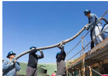
Concrete from ready mix truck delivered through pump and hoses; all hands on deck to manage hoses heavy with concrete
