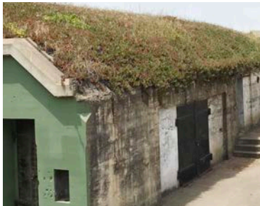
Before: Deteriorated condition, visitor safety compromised
