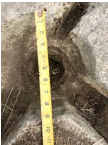
Condition assessment revealed non-functioning drainage pipe
