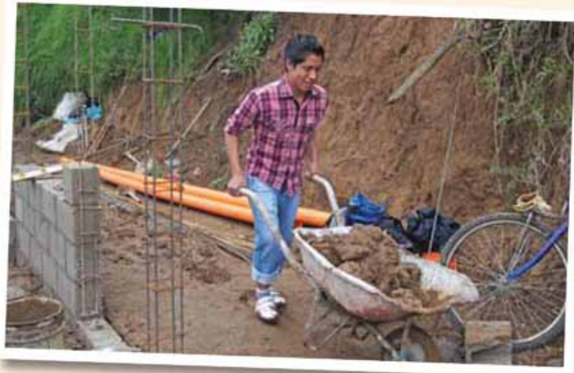
A leader in training helps to build a home for a destitute family.
