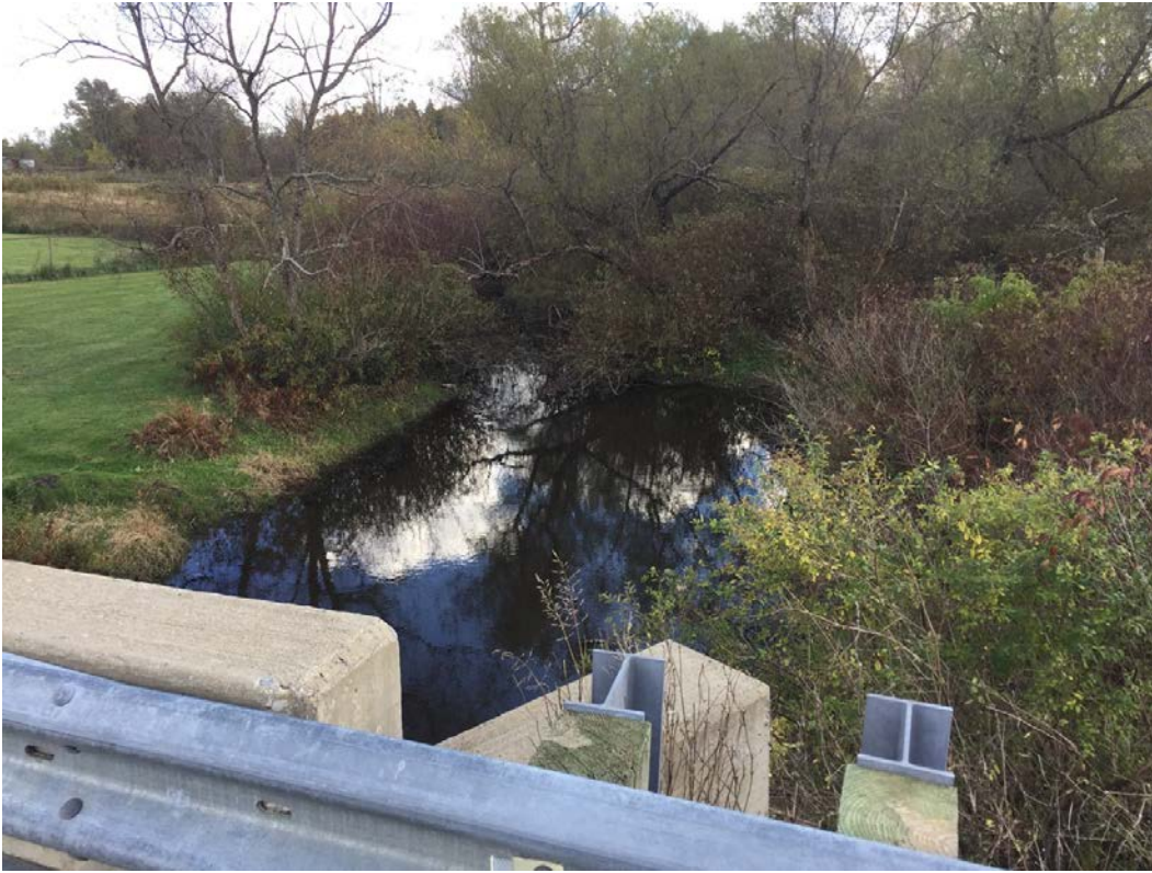
Figure 51. Elk Creek, looking downstream at Greenlee Road bridge, northwest of the Marsh Site.
