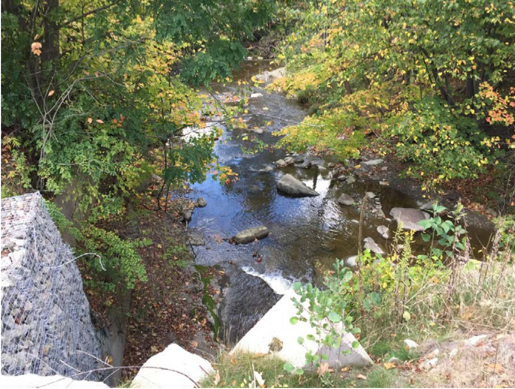
Figure 53. Elk Creek crossing under Oliver Road, steep-sided gorge; bridge supported by gabions.
