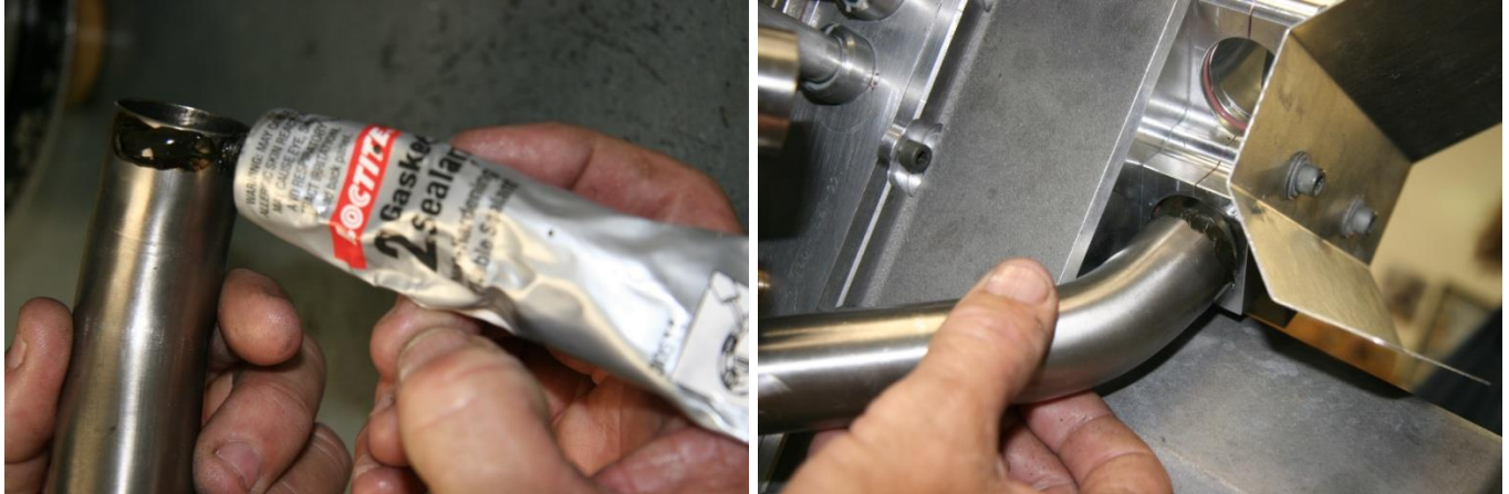
Figure 199 – Fitting Induction Pipes to Plenum Chamber
