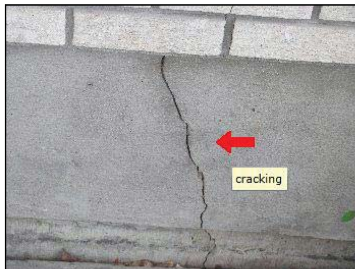
9. Typical minor cracks
