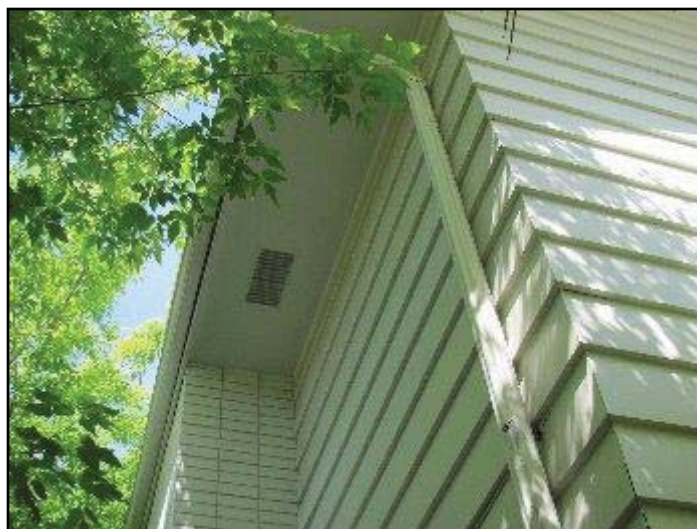
2. Missing, loose or torn
