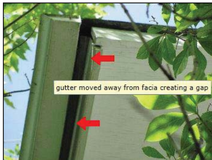
4. Loose or damaged
