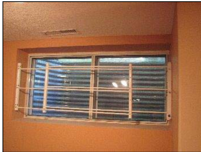
16. Burglar bars not operable without tools
