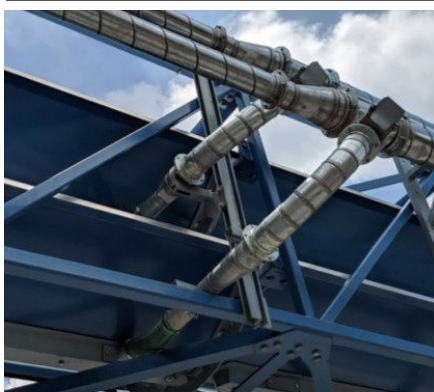
Air Supply Ducting
