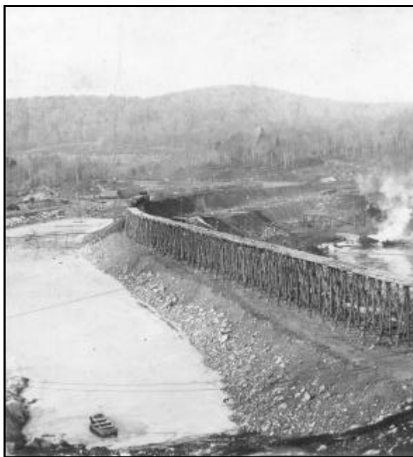
This trestle was built along the designated path of the dam. Trains hauled and dumped loads of earth along this route, which buried the trestle within the earthen dam.
