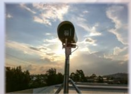
LightPointe HyBridge LXR-5 wireless bridges installed by Star-Tech
