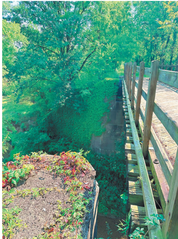
Photo 8 Beaver Creek Railing and Drop Off
