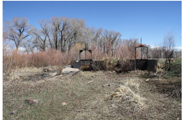
Headgate, diversion dam, and return gate
