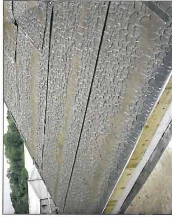
Wrinkled rubberized underlayment due to overexposure.
