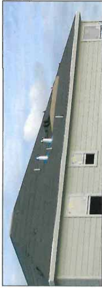
Felt underlayment displaced by wind.
