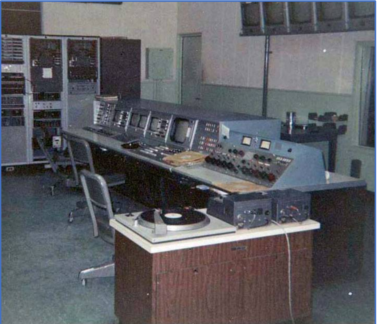
The TV Control Room
