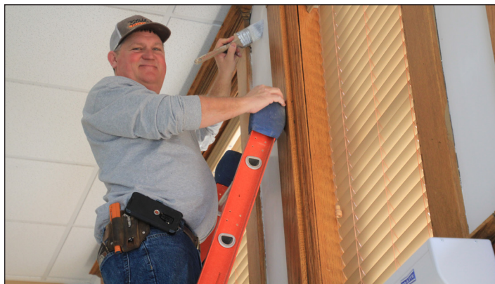
Brett Stahl is priming in the gallery after the repairs are completed. LOOKING GOOD even with 1 coat left to go!
