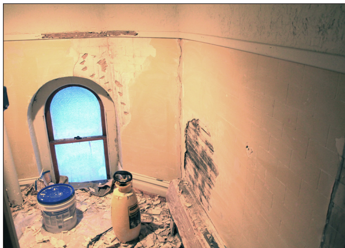
We haven't forgotten the bathroom. This room has received a new coat of repairs, paint and a little tweaking to hopefully accommodate a wheel chair. It is not completely done yet.
