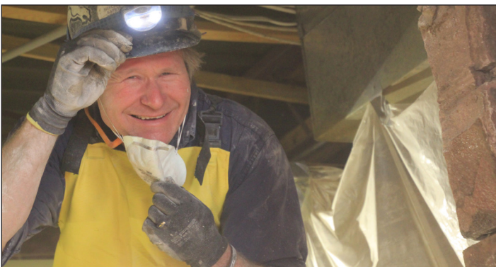
Widening the door between the Corn Palace Room and the Gallery. This is being done for ADA compliance. The “man with the saw” Doug Kaemingk smiles as he takes a break from working on the door.
