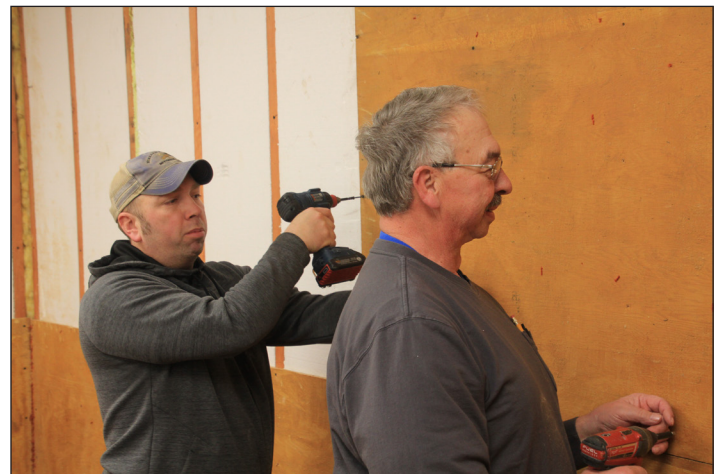
Ben Letcher and Bruce Huebner from Mueller Lumber replacing the plywood in the Corn Palace Room.
