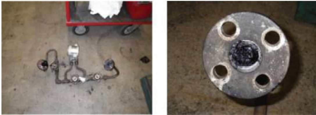
Fig. 5 : DP Assembly Removed (Left) and Impulse Lines Blocked (Right)
