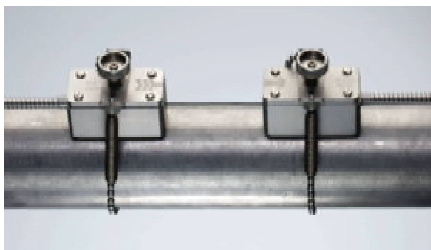
Fig. 1: Two clamp-on transducers on a steel pipe
