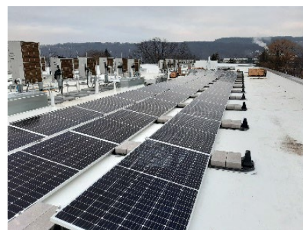
Solar Array at Glen Lakes Apartments
