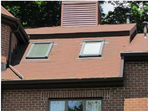
Partial shingle replacements and lifted shingles at Building 2
