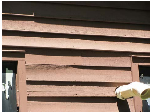
Warped wood siding
