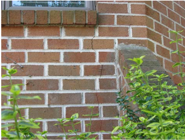
Masonry crack at Unit 1
