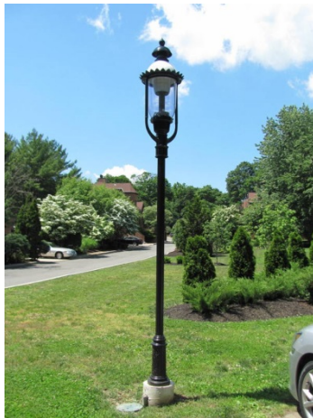
Light pole and fixture
