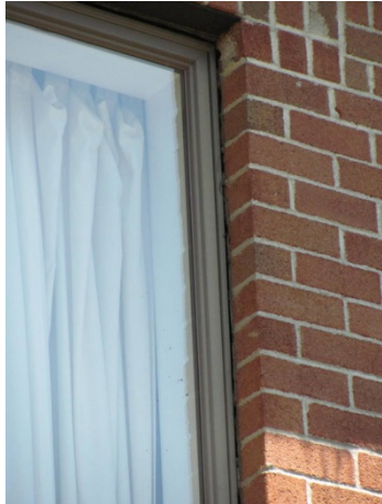
Adhesion failure at sealant
