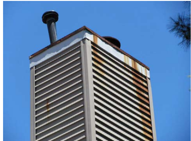
Loose chimney cap and significant rust at Building 1
