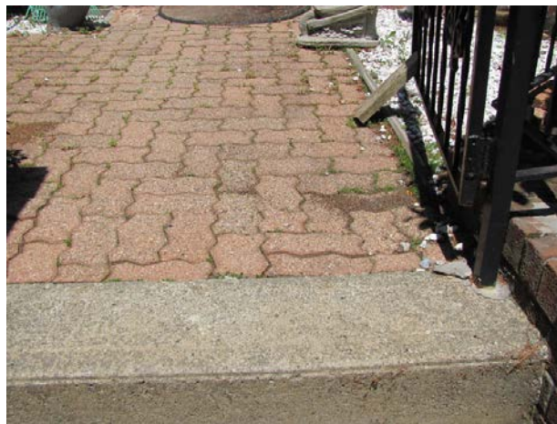
Settlement at walkway
