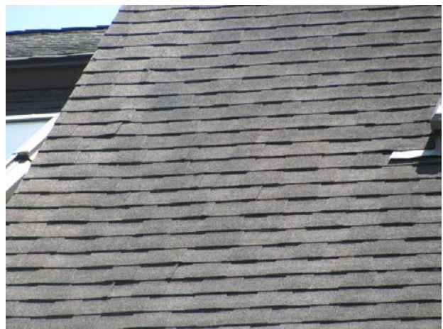
Weathering evident at shingles at Building 3
