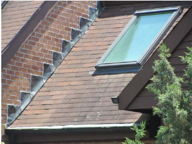
Cupped and weathered shingles at Building 1
