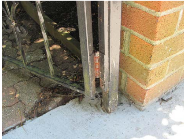
Rust at post and hinge
