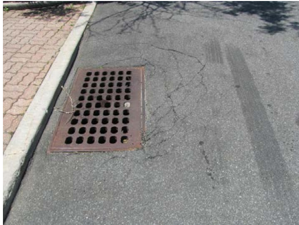
Alligator cracks adjacent to catch basin
