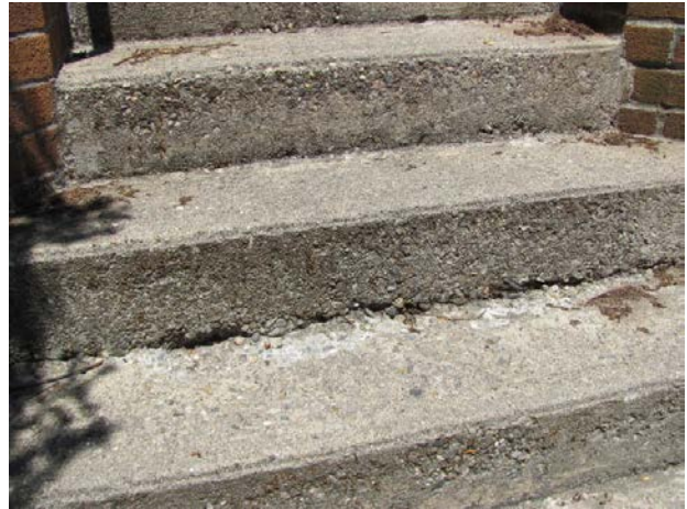
Spalled concrete stairs at Unit 36
