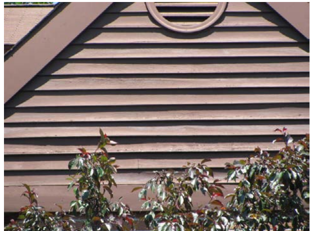
Faded paint finish at south facing elevation
