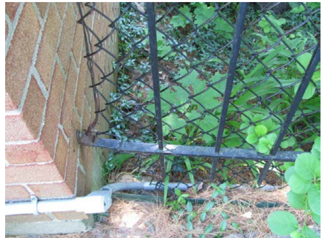
Rust at bottom fastener
