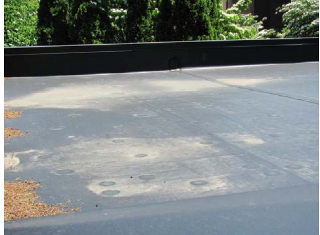
Standing water evident at garage for Units 27 and 28
