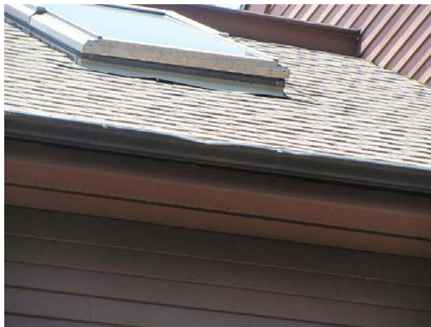
Dented gutter at Building 3
