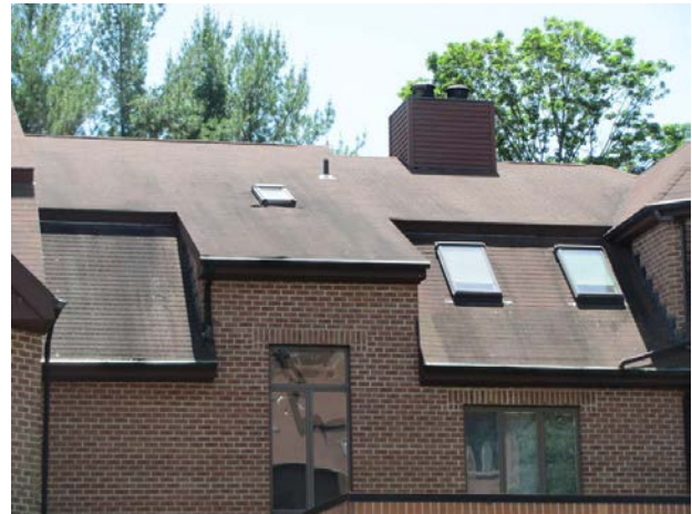
Weathered shingles at older roofs at Building 1
