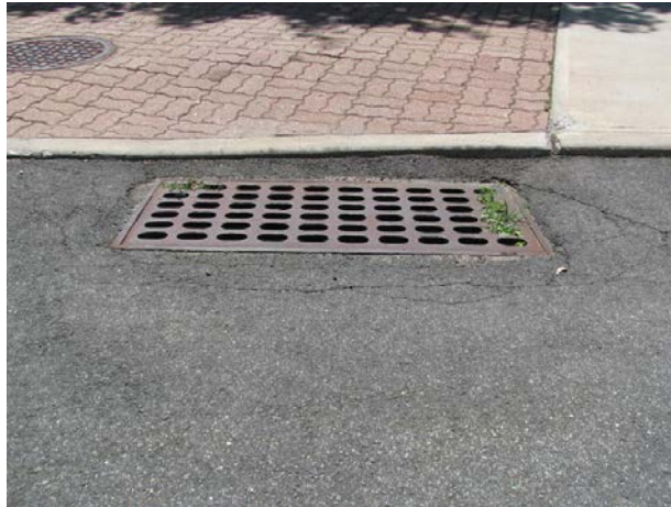
Settlement at catch basin
