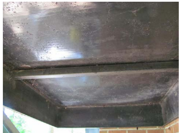
Balcony underside, note rust at ends
