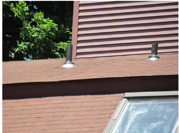
Sheathing deflection evident at Building 2
