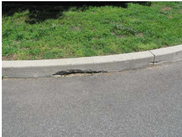
Spalled concrete curb
