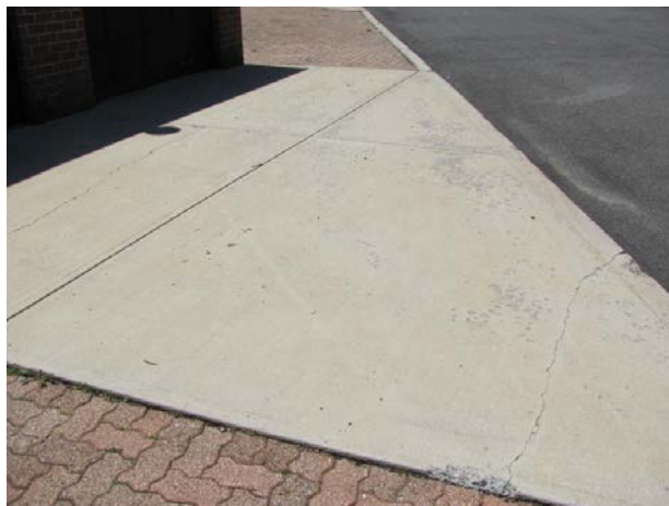
Cracks and spalls at Units 3 and 4
