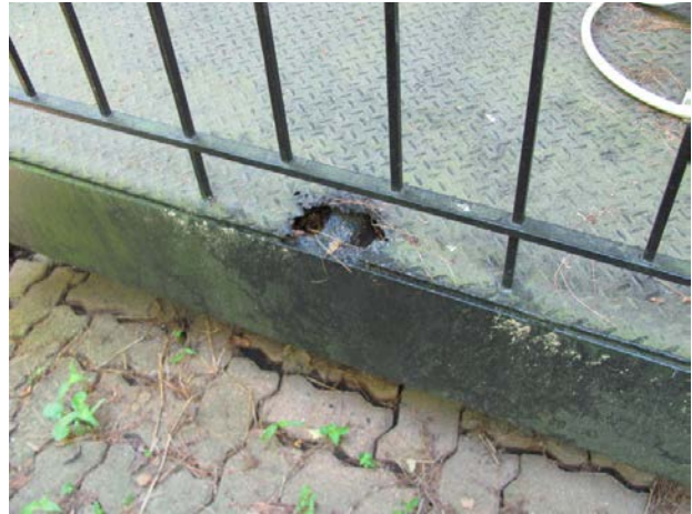
Corroded metal at Building 2
