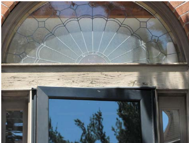
Chipped paint at wood trim
