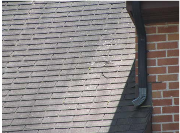
Granular loss and cracked shingles at Unit 2 at Building 1
