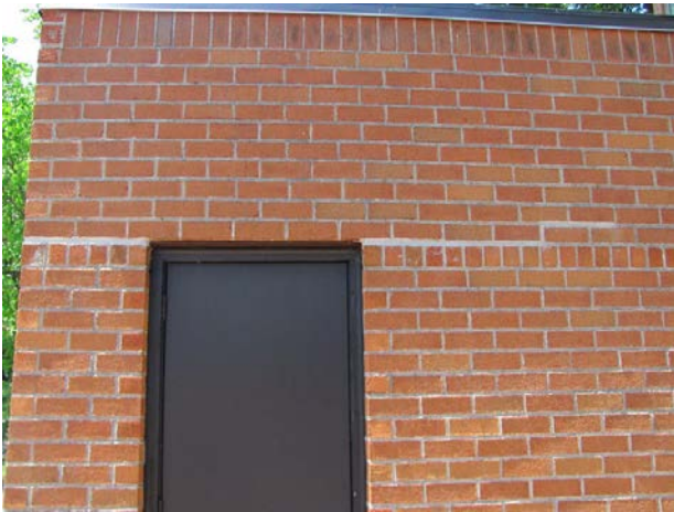
Recent mortar repairs at garage
