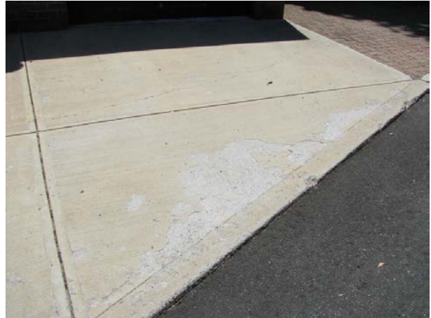
Concrete spalls at Units 1 and 2
