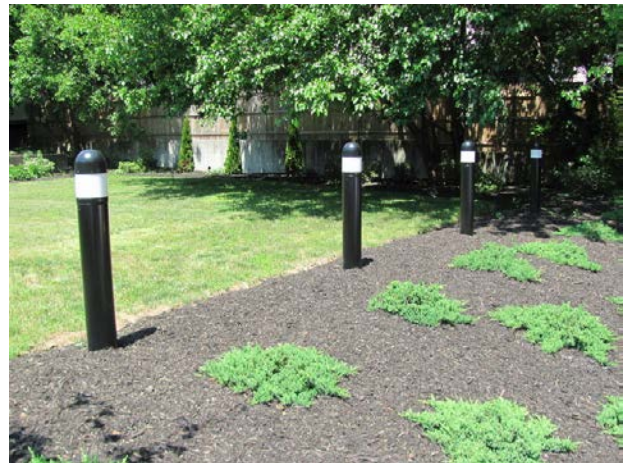
Bollard light fixtures
