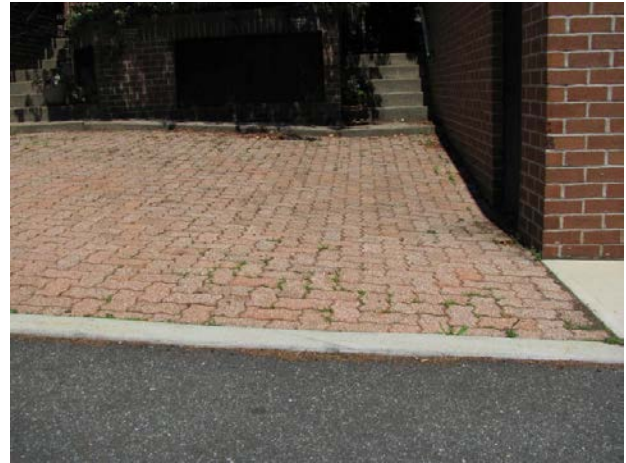
Settlement evident and organic growth at Unit 34
