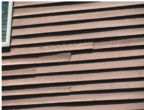
Weathering near joints/fasteners
