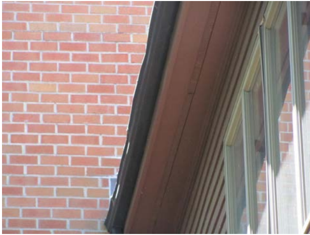
Dented aluminum gutter at Building 1
