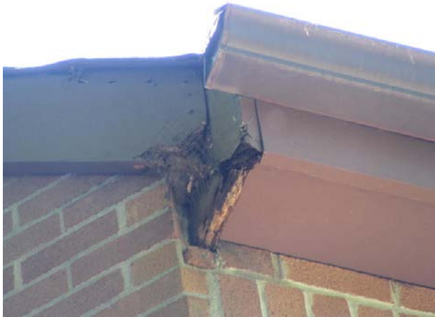
Wood rot at soffit and fascia
