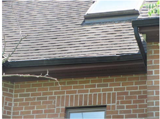
Deflected gutter at Building 3
