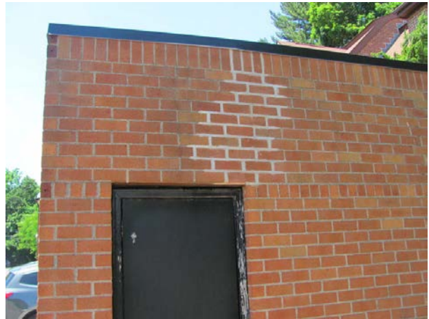
Recent mortar repairs at garage
