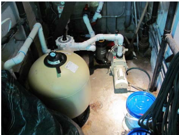
Pool mechanical equipment
