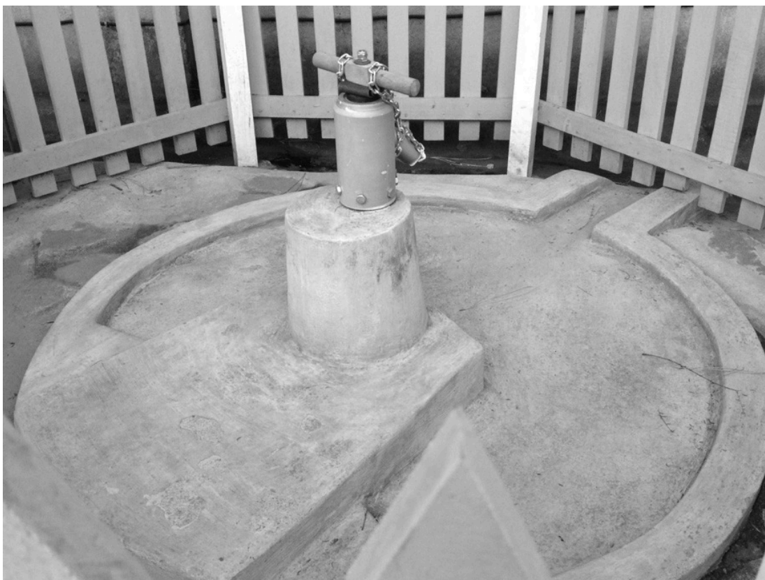
Figure 9. Completed well with Canzee, apron and drainage (note: the chain seen in the photo was not used on project pumps). Photo by author
